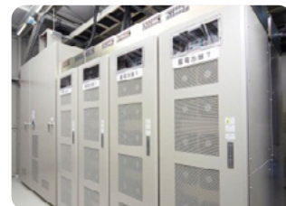
Regenerative power storage device
