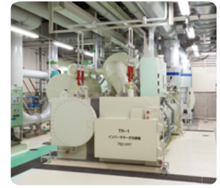
Kinshicho Heat Supply Facility
