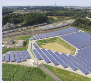
Tobu Takayanagi Solar Power Plant (Tobu Energy Management)
