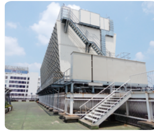
Nishi-Ikebukuro Heat Supply Facility
