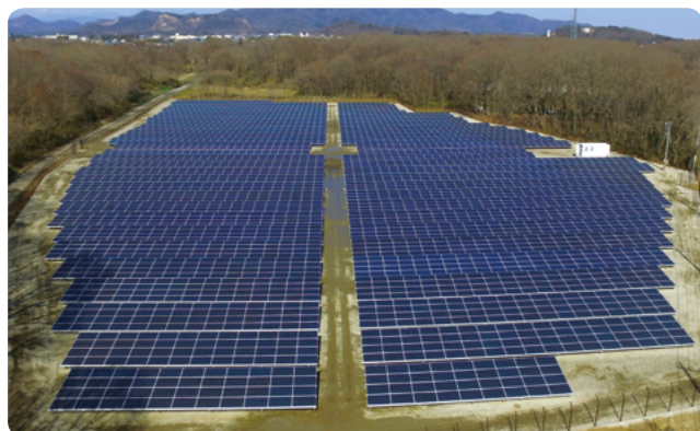
Tobu Iwafune Solar Power Plant
