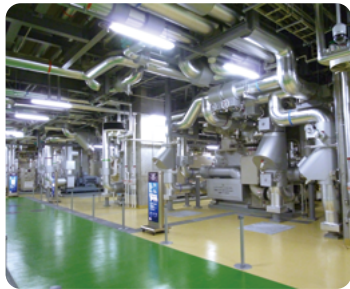
Major heat supply facilities in the TOKYO SKYTREE area
