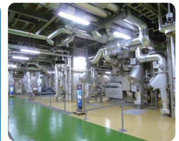
Heat supply facilities in the TOKYO SKYTREE area
