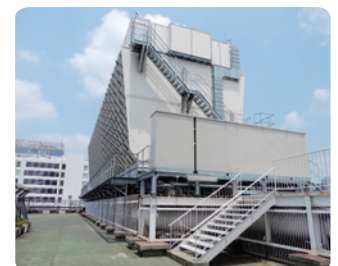
Nishi-Ikebukuro Heating & Cooling Supply (Sub-plant)
