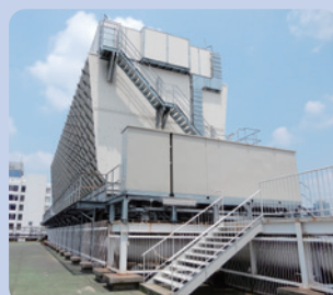
Heat supply facility (sub-plant) (Nishi-Ikebukuro Heating & Cooling Supply)
