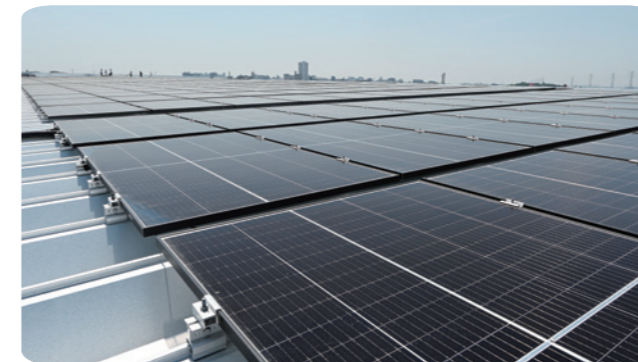
Solar panels installed on the roof of a distribution warehouse
