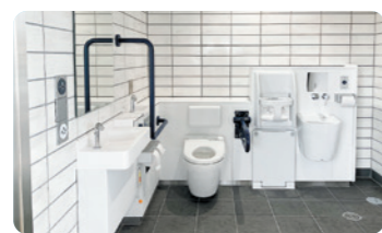
Barrier-free toilet (Omochanomachi Station)
