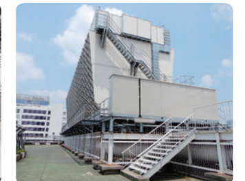
Nishi-Ikebukuro Heating & Cooling Supply (Sub-plant)
