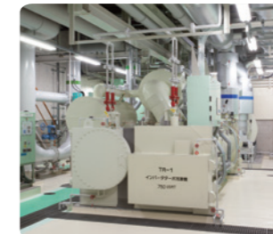
Kinshicho Heating & Cooling Supply (Plant)
