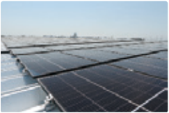
A Tobu Shoji solar power generating station
